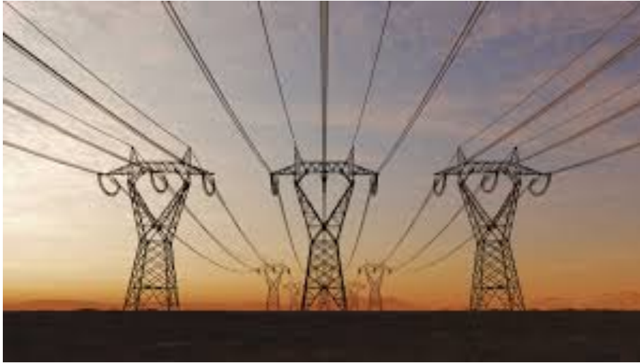
240 KV Transmission lines
